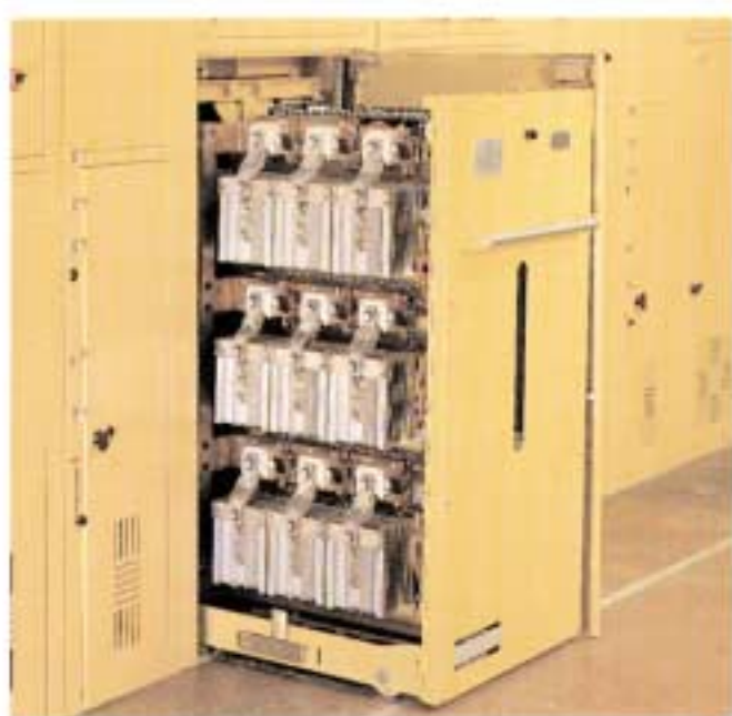
Rectifier cell for Genoa subway
