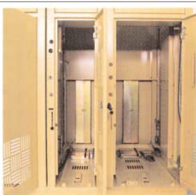
Interior of circuit breaker and connector cells
