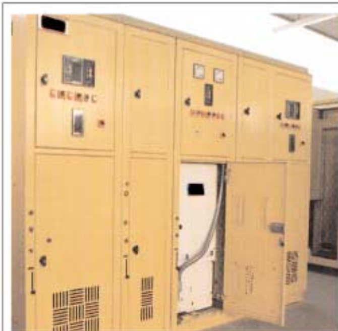
The circuit breaker cell
