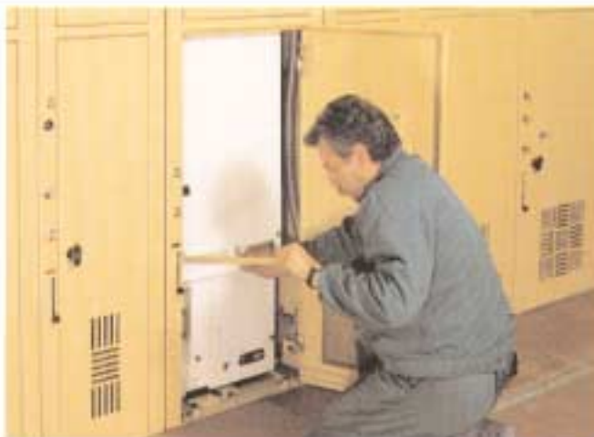
Operation for the circuit breaker insertion
